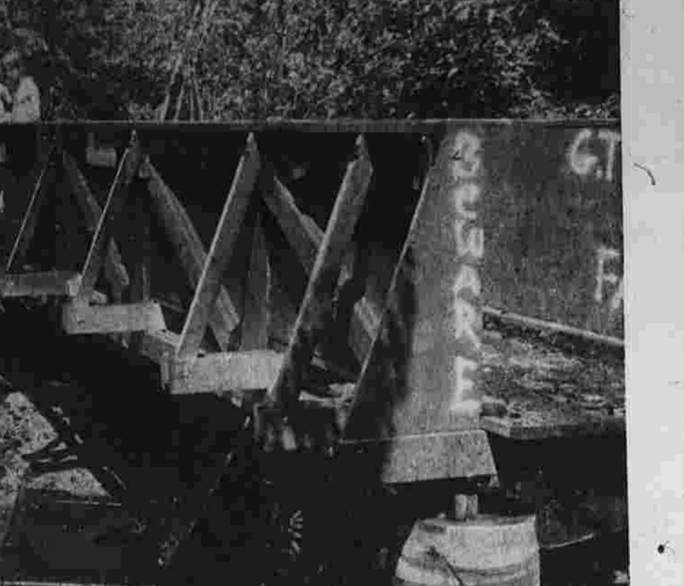
A suspicious Tuesday afternoon fire badly damaged the recently installed footbridge over Lydall Brook below the Salter's Pond dam in Manchester. Today the bridge was barricaded and officials said the structural damage caused by the fire cannot be repaired. (Herald photo by Pinto)
